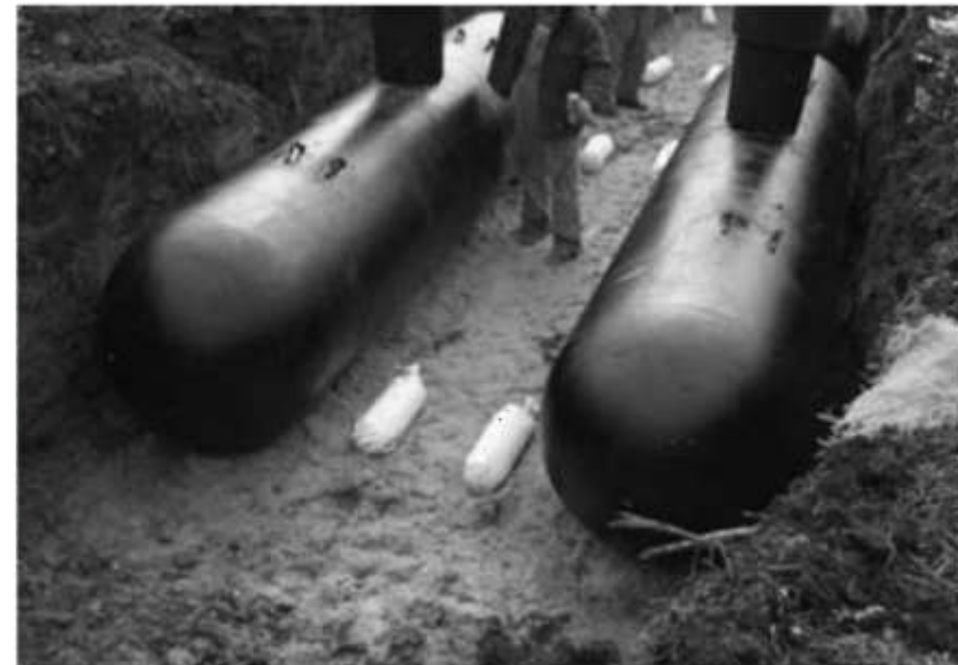
EXHIBIT 6.17 Installation of Two Underground Tanks, Showing Placement of Anodes (Courtesy of H&H Gas)
